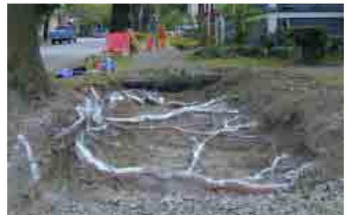
Fig. 1.4 Surface rooting of trees growing in compacted soils
